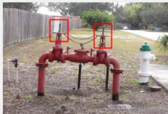
A backflow preventer with two outside screw and yoke (OS&Y) valves is in the open position since the valve stem is visible (highlighted by red boxes). When an OS&Y valve is shut, the stem is not visible.
